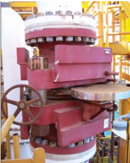
Fig. 6 – 20 inch ASME 600# Offshore Cam-Set – Gulf of Mexico
