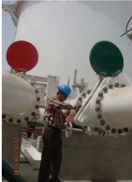
Fig. 1 – Cam-Sets installed in a tank farm in UAE
