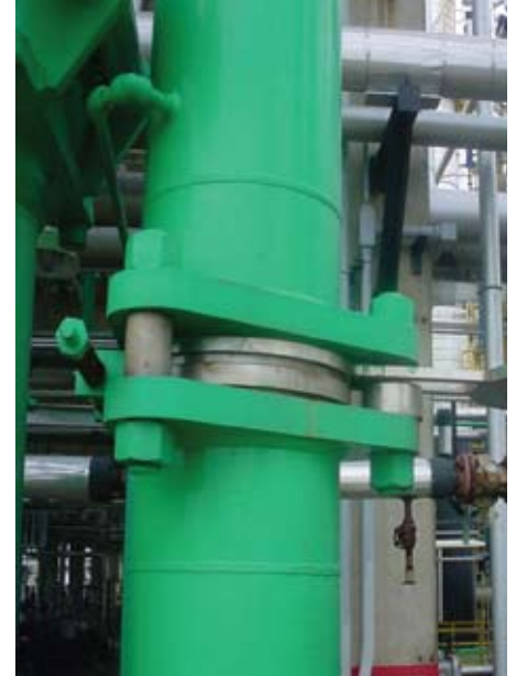
Fig. 2– Cam-Sets installed in Hydrotreating plant in Brasil
